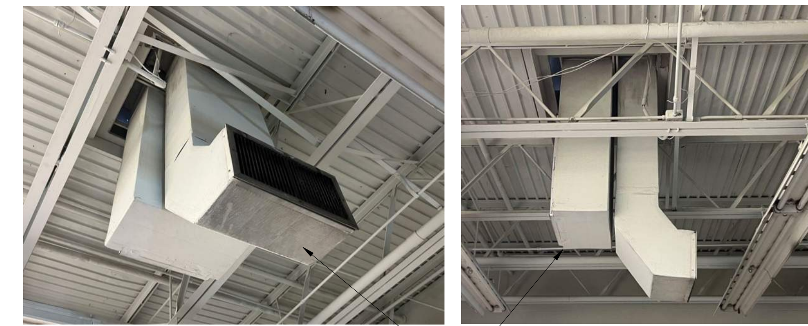
FOR RTU-6 AND RTU-7, REMOVE EXISTING DUCTWORK AND PROVIDE NEW CONCENTRIC SUPPLY AND RETURN DROPPING DOWN BETWEEN BAR JOISTS
