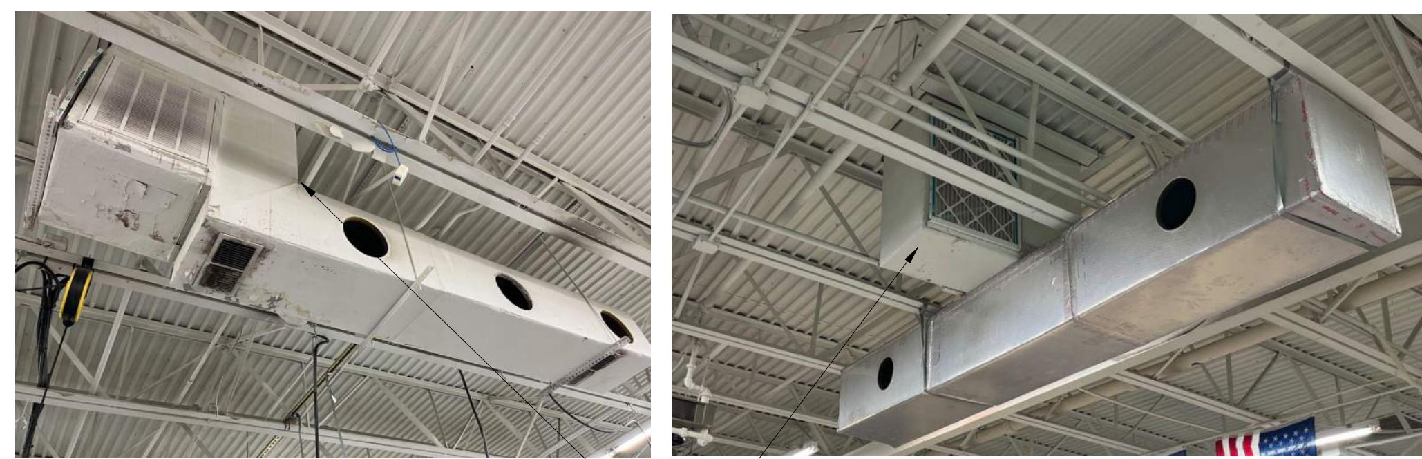
FOR RTU-1 AND RTU-3, REMOVE WOOD FRAMING AND EXISTING DUCTWORK AND PROVIDE NEW CONCENTRIC SUPPLY AND RETURN DROPPING DOWN BETWEEN BAR JOISTS
