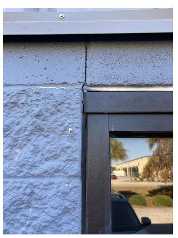
EAST ELEVATION - SEALANT NEEDED AT EXISTING STOREFRONT
